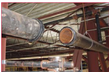
Tuberculation in the aqueous film-forming foam fire-suppression deluge system was one reason for system failures and false alarms.
